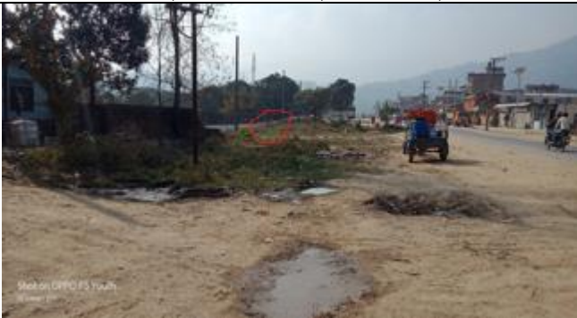
Public Toilet construction area (103 sqm) , ward 4 Tamaghat Bazar, Beyond ROW, 25 m away from central line
